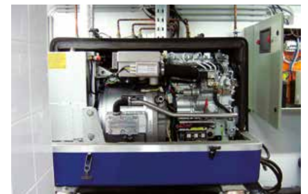
This three-phase Panda is installed in a basement. Main fuses, panel and radiator control are fitted in an electrical cabinet.
