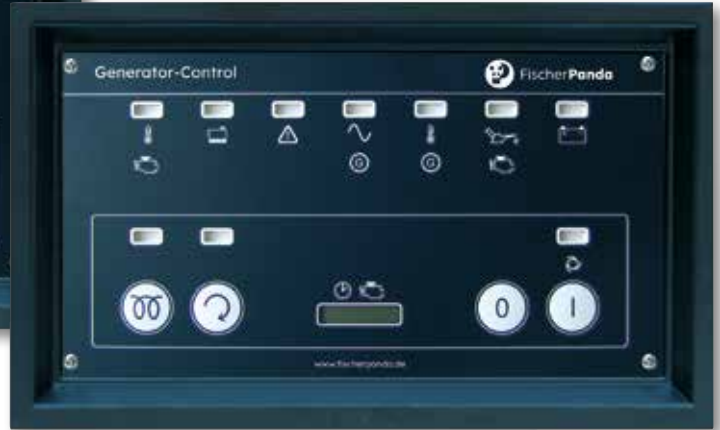
Panda P6 Plus Remote Control Panel 2
